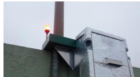
Fig. 2. Current sensors installed on the lightning rods of buildings P1 and P2 (upper picture) and detail of the installation (lower picture).
