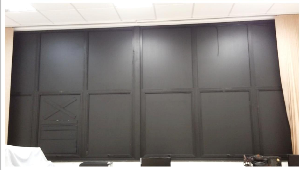
Figure 25: Darkening of laboratory windows of the room 4 at the ground floor of the INPE's Building CEA II.
