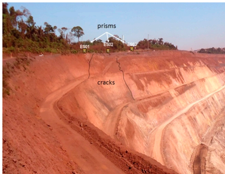
Figure 9. Presence of cracks on the pit benches related to the SW sector of the N5W mine and prisms locations.
