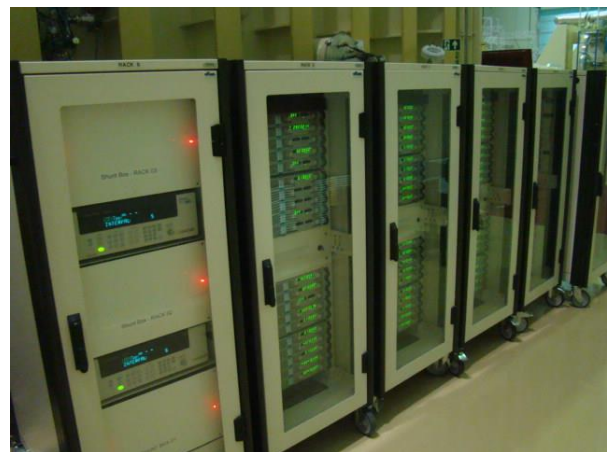
Fig. 5 - Electrical Power Supply System to spacecraft and set-up heaters
