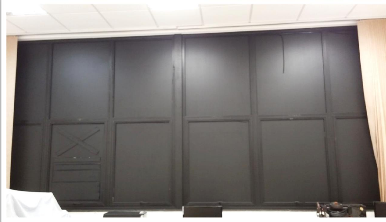
Figure 25: Darkening of laboratory windows of the room 4 at the ground floor of the INPE's Building CEA II.
